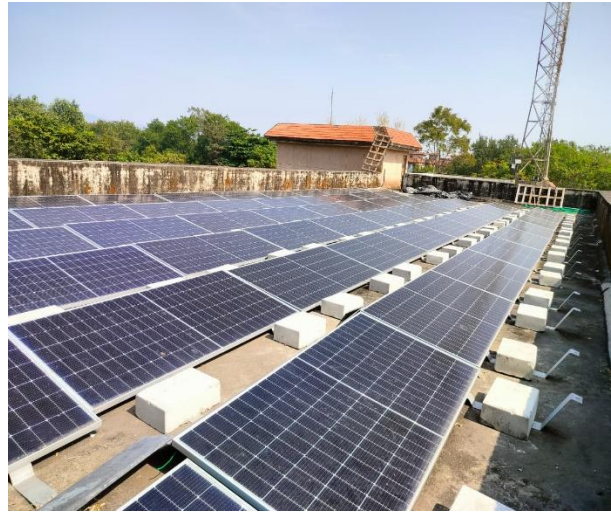
2) Mangal Bhavan 30 KWp
