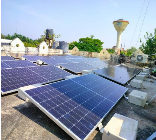
4) Shopping Complex – 30 KWp
